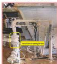
Manual Valve before the Installation
