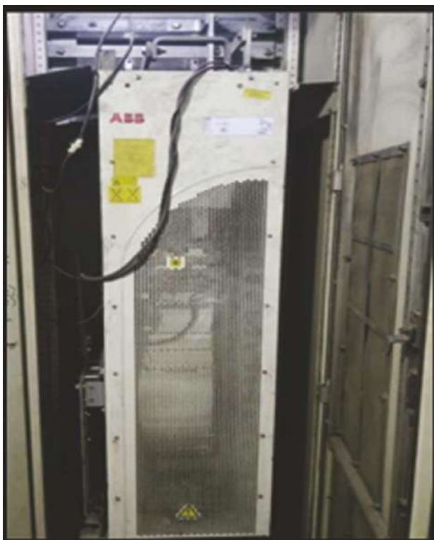
REDUNDANT BACKUP DRIVE
