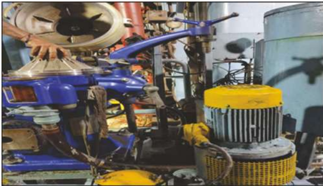
Actual Finishing Mill J-11 lubrication system comprising feed pump, oil separator and associated piping
