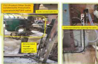
Pneumatic ON/OFF valve Installation
