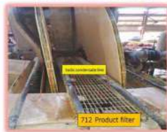
Normal Sodic Condensate Line in Product filter
